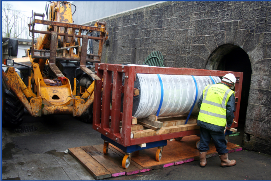
Replacement Pillar arrives and workmen begin to bring it into the Cathedral via the Crypt.
