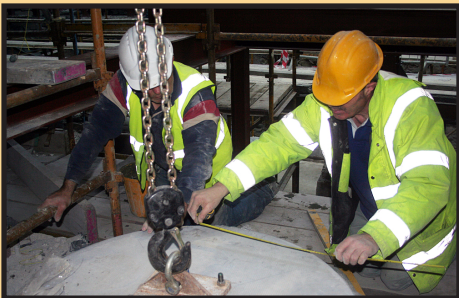
Pillar foundation stone being measured as workmen begin the process of setting it in place.
